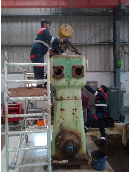
Image 1: The 30-year-old compressor had been out of service for a considerable time.
