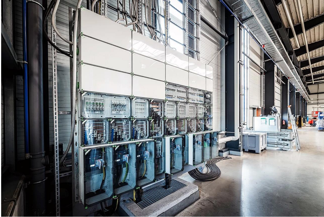
Image 2: The modular Spelsberg GTi series installed on-site, offering customizable distribution without facility construction.
