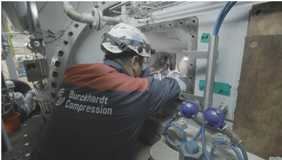
Image 3: Burckhardt Compression can deploy experienced personnel and their equipment to support planned maintenance in shipyards, ports or at sea.
