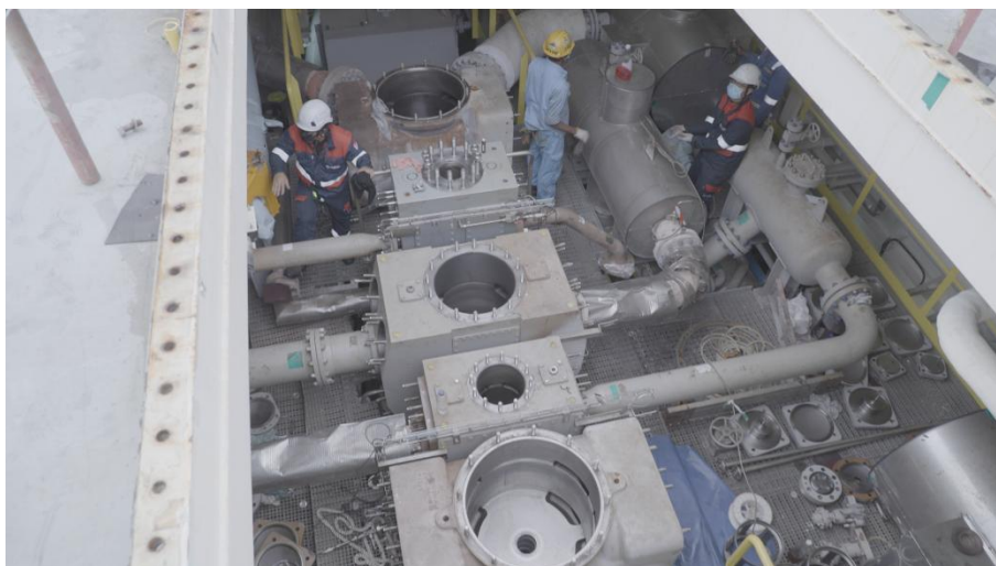
Image 4: Coordinated compressor maintenance in dry-dock is crucial for long-term efficiency and reliability.
