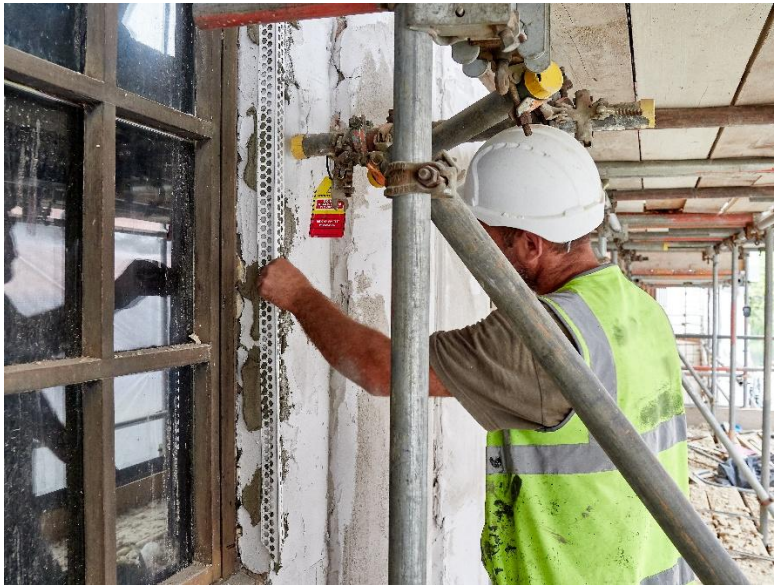
Image 4: Over 2,500 linear metres of Renderplas PVCu beads were installed to ensure crisp architectural detailing.
