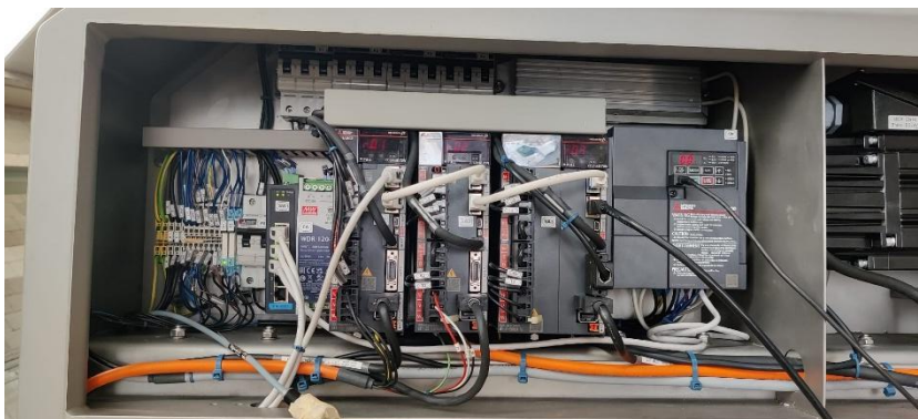
Image 4: Adopting CC-Link IE TSN has reduced wiring and integration complexity, making commissioning faster and easier to support.
