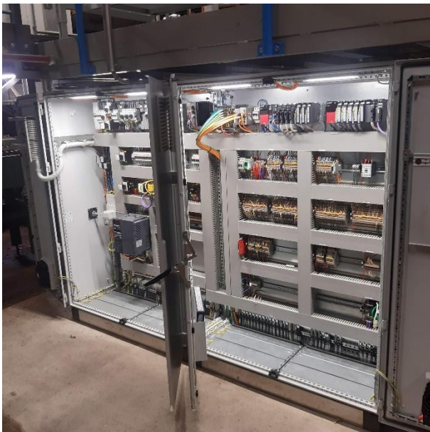
Image 2: Moving to CC-Link IE Field brought benefits including improved fault diagnostics, a more flexible wiring structure, and simpler hardware configurations.
