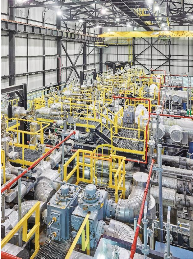
Image 1: A typical terminal equipped with LNG compressors
