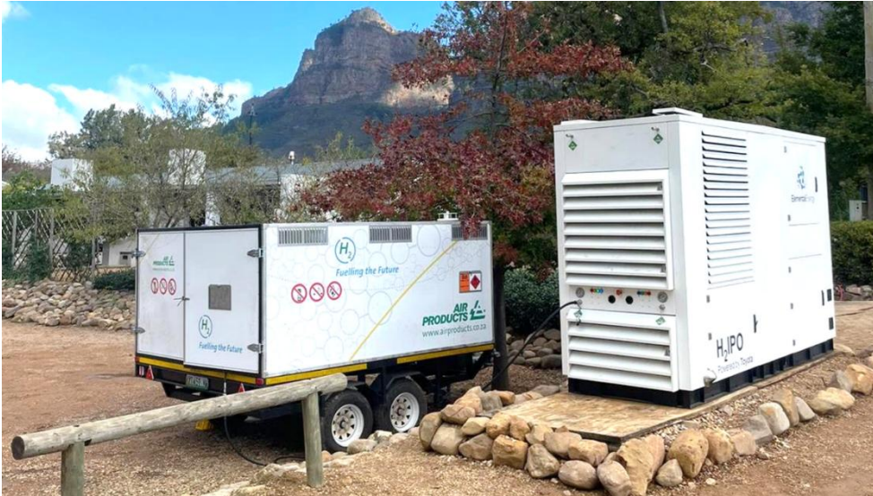
Image 1: The self-contained microgrid provides reliable and green power for remote locations.
