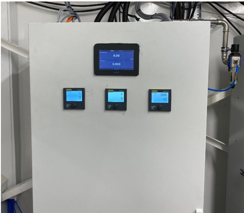
Image 2: The information displays are in the control room while the flowmeters are in an ATEX Zone 2 hazardous area.
