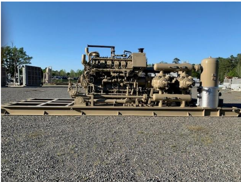
Image 2: Compressors in more remote locations provide additional challenges.
