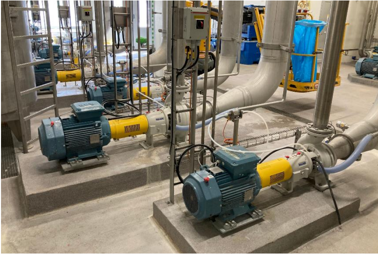
Image 3: A-LM pump units on fiber separation
