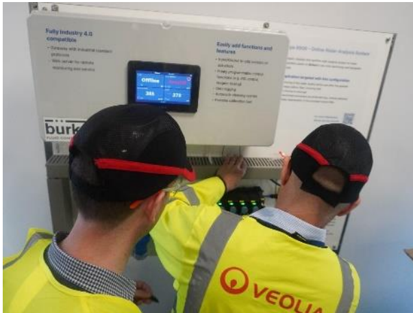
Image 1: Installation of the compact Online Water Analysis System was a simple process
