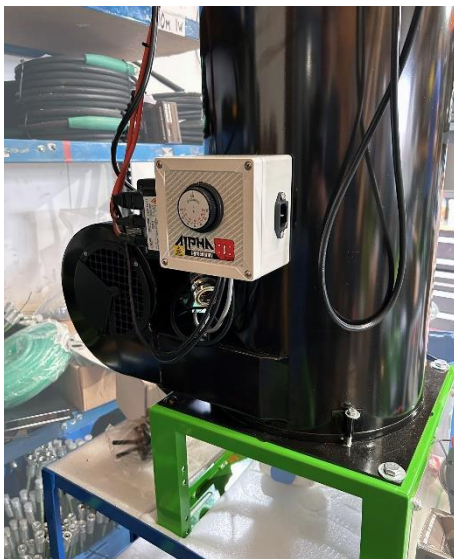
Image 2: Spelsberg custom heavy-duty junction boxes to house the thermostats for hot-water washing machines from Precious Washers Stafford Ltd.
