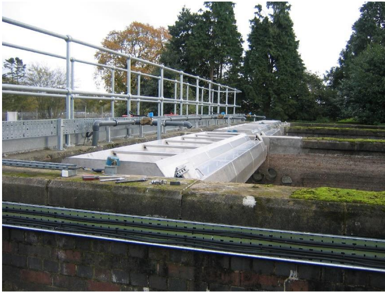
Image 3: The works include the design, installation, maintenance and testing of mechanical assets at water and wastewater facilities
