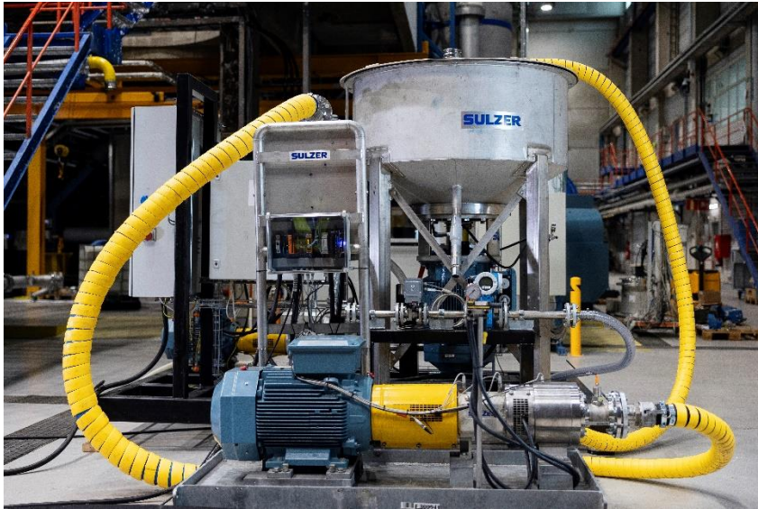
Image 1: MCE test loop at Sulzer's development centre.
