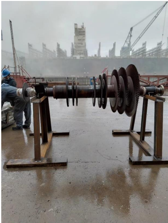
Image 1: An 18-year-old 5 MW steam turbine installed on a 98'000-ton container ship suffered damages due to operational wear and tear.
