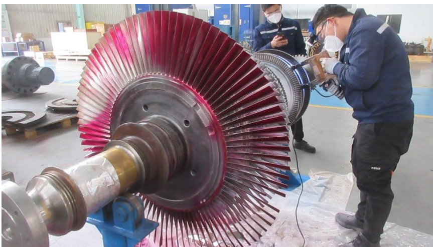
Image 2: Sulzer teams in China, Singapore and Indonesia collaborated to determine the best approach for repair.
