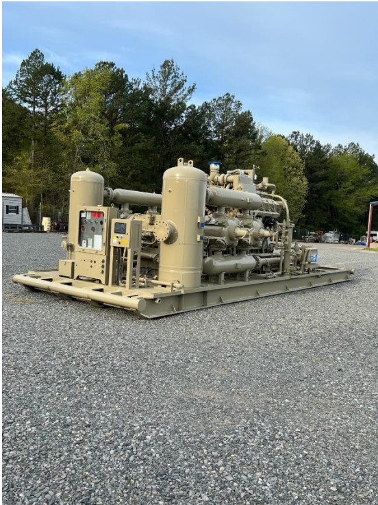
Image 3: Compressors on skids, prepped for delivery
