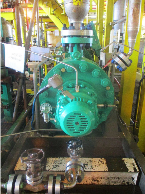
Image 3: Following the retrofit, the MTBF for the pumps was increased from 12 to 48 months.
