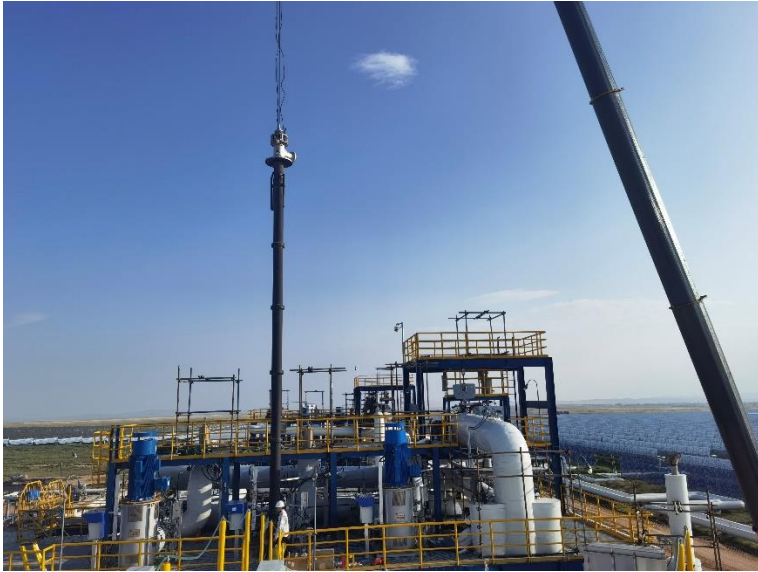
Image 1: A lithium carbonate manufacturing plant in Asia has selected Sulzer to supply pumps for its molten salts energy storage system.
