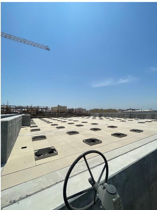
Image 2: The 160 new DynaSand filters will double the capacity of the plant
