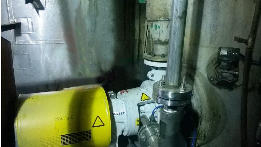
Image 1: Sulzer's MCE pump at the site
