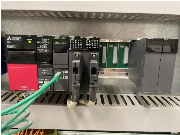
Image 5: To control the 19 VSDs, Profile Developments selected Mitsubishi Electric's iQ-R series PLC. [Source: Mitsubishi Electric Ireland]
