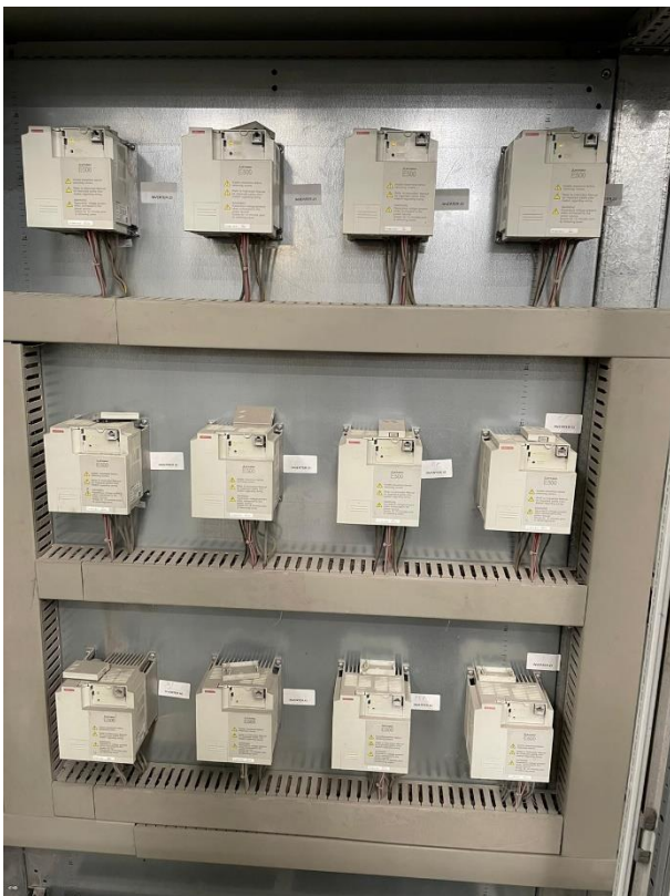
Image 2: Profile Developments wanted to build a new panel gluing unit to ramp up productivity. [Source: Mitsubishi Electric Ireland]
