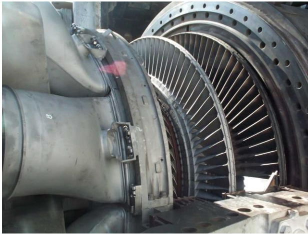
Image 1: To meet the new emissions standard, it was clear the turbine required a retrofit solution.
