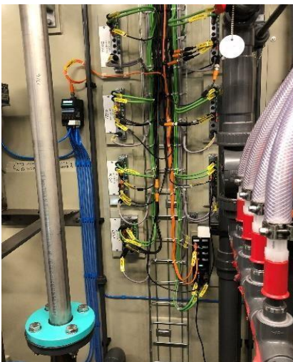
Image 2: The 8653 used in these pilot plants are IO-Link enabled and do not require Communicator to transfer settings.
