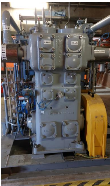
Image 2: Refurbished compressor skid installed at customer's plant.
