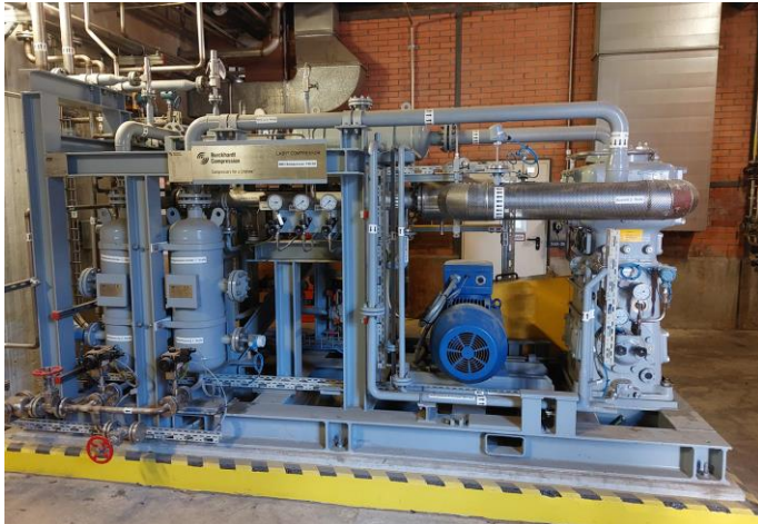
Image 1: Laby® compressor test run in accordance with Burckhardt Compression regulations.
