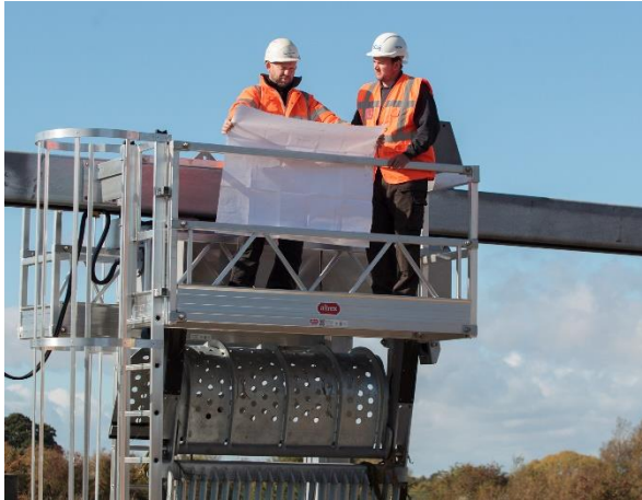
Image 1: ECS can provide comprehensive maintenance services for water control assets, pump equipment, and structures.
