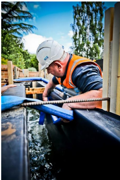
Image 2: The company has expertise in covering pumps, sluice gates, and water control structures
