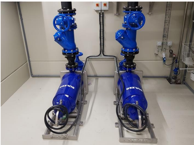
Image 2: The XFP pumps working in a duty/standby arrangement, give the station a capacity of 25 liters per second.
