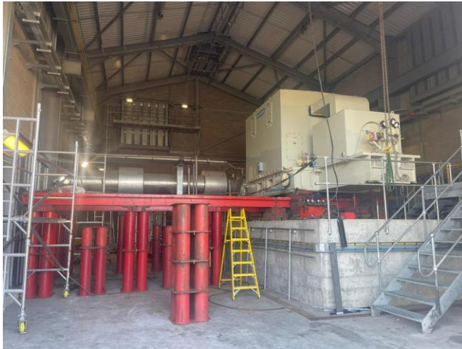
Image 1: At gas booster stations, motor driven compressors are used to ensure the distribution of gas to where it is needed
