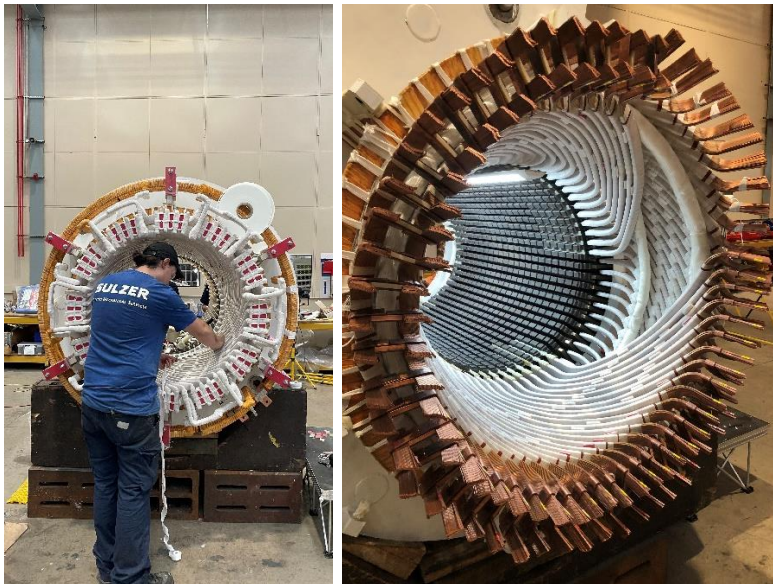
Image 2 + 3: The design and installation of replacement RTDs necessitated a complete rewind, testing, reinstallation and commissioning
